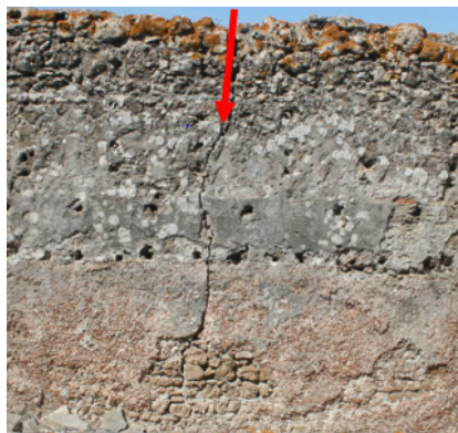
Fig. 4: Vertical fissure crossing a wall in the large western baths (Author's photo 11/10/2022)
