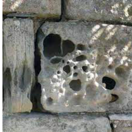
Fig. 3: Intense alveolization (Variable shape and size cavities) (Author's photo 11/10/2023)
