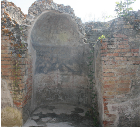
Fig. 2: Thermal bath wall with frescoes showing signs of capillary rise (Author's photo 11/10/2022)
